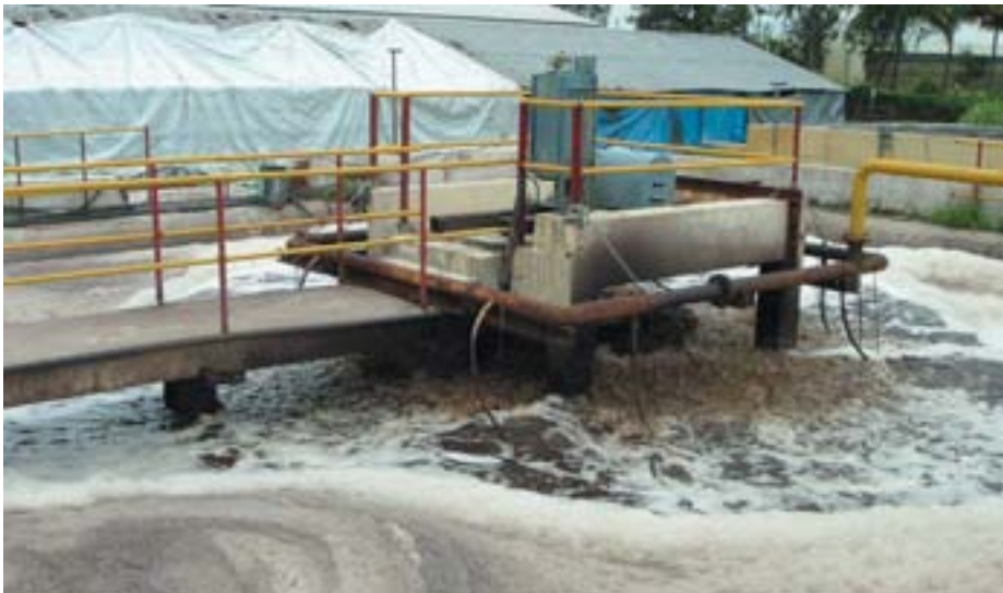
Effluent treatment plant at SSCL, Berigai.
